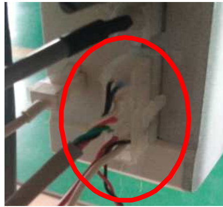
Fig.20 After the 373D sensor is installed
