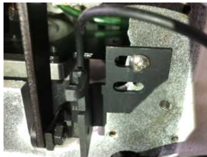
Fig. (11) After Button Sender Sensor Installation
