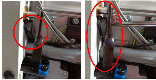
Fig. (13) After the Sensor Installation Fig. (14) After the Sensor Installation
